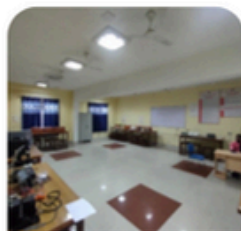
Power Electronics Lab
